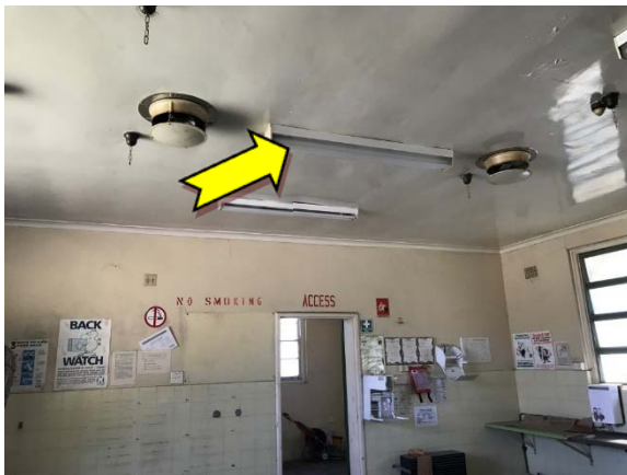
Photo 9. Interior, throughout, double tubed fluorescent light fitting – suspected PCB-containing capacitor.
