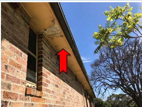
Photo 5. Exterior, throughout, eaves – suspected asbestos-containing fibre cement sheeting and suspected lead-containing cream upper paint systems.
