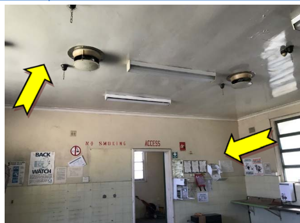
Photo 12. Interior, throughout, walls and ceiling – suspected lead-containing yellow and white upper coloured paint systems.
