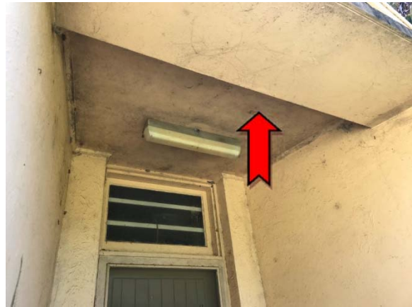
Photo 4. Exterior, north elevation, awning – suspected asbestos-containing fibre cement sheeting.
