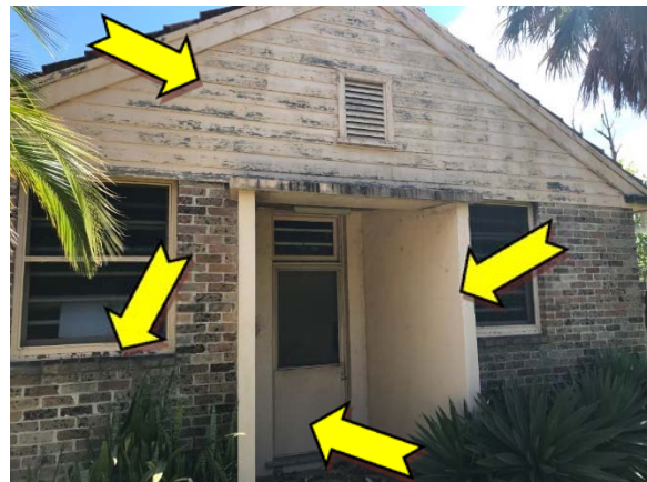
Photo 10. Exterior, throughout, window frames, doors, gable and features – suspected lead-containing cream upper coloured paint systems.
