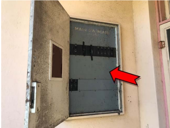
Photo 7. Exterior, south-west elevation, electrical backing board – suspected asbestos-containing bituminous backing board.
