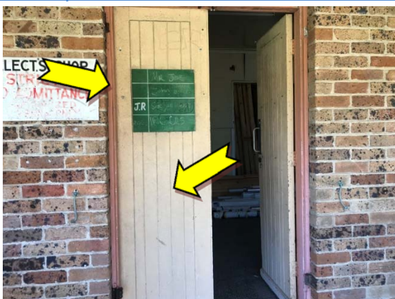
Photo 11. Exterior, throughout door and door frames – suspected lead-containing orange and cream upper coloured paint systems.
