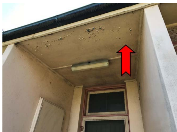
Photo 6. Exterior, south-west elevation, awning – suspected asbestos-containing fibre cement sheeting.
