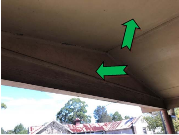
Photo 1. Exterior, south elevation, main entrance, awning and fascia – non asbestos-containing fibre cement sheeting.
